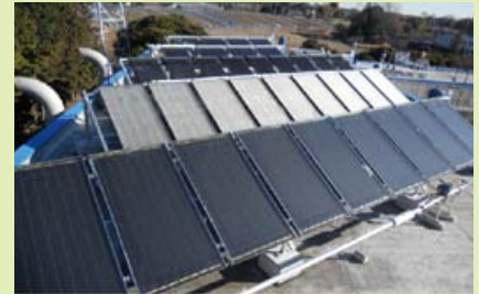
A solar thermal collection panel at the Hibiya Engineering Technology Research Center
