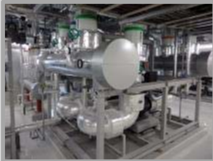
Air conditioning machinery room
