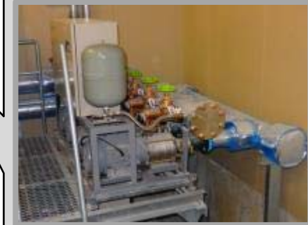
Water supply feed pump
