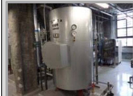
Hot water tank
