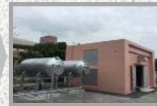
Gas holder and control room
