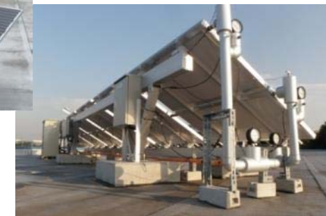
Solar heat collection units are placed under the photovoltaic panels.
