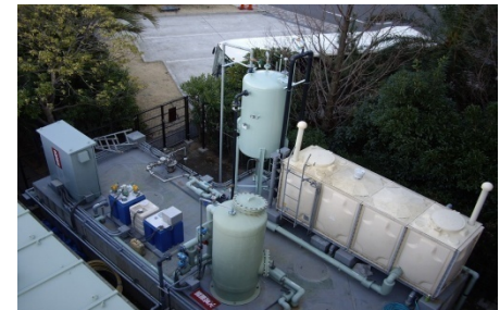
Cogeneration system using natural gas
