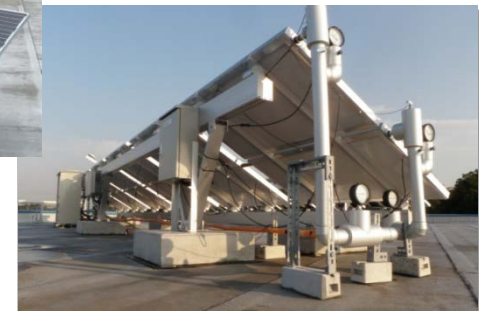
Solar heat collection units are placed under the photovoltaic panels.
