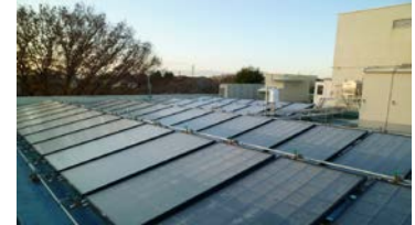
Solar thermal system
