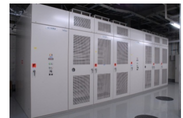
Building electrical system
