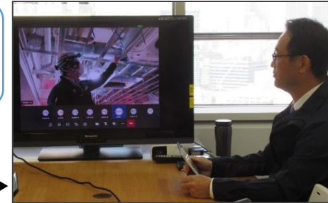
A remote site inspection being made using a wearable camera and a communication app ▶
