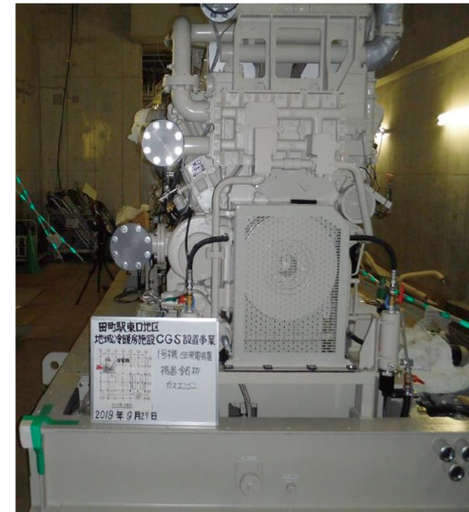
Upgraded gas engine
