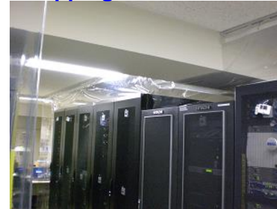
Installed under a ceiling beam
