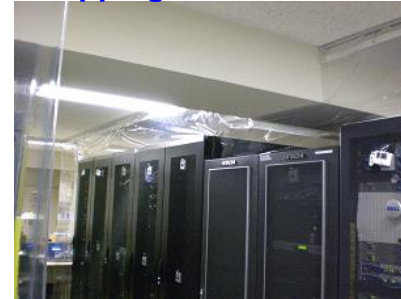
Installed under a ceiling beam
