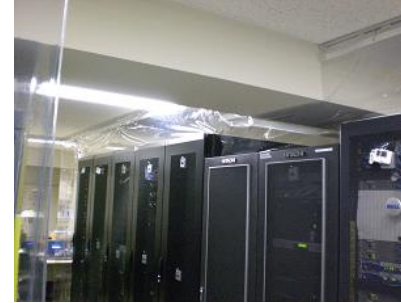
Installed under a ceiling beam
