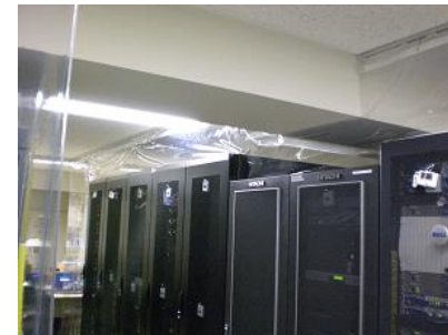
Installed under a ceiling beam
