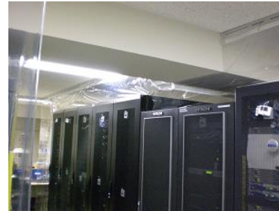
Installed under a ceiling beam
