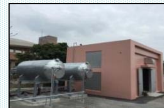
Gas tank/Control room
