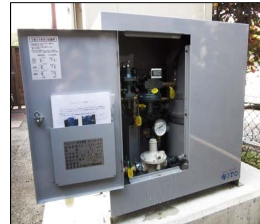
[A cogeneration system that uses LP gas (control section)]
