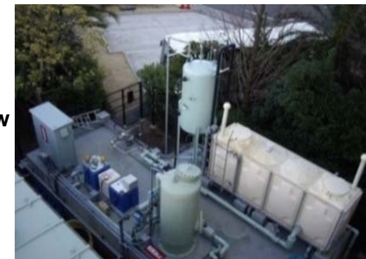
Natural gas cogeneration system
