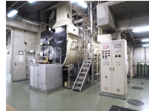
Heat generation equipment
