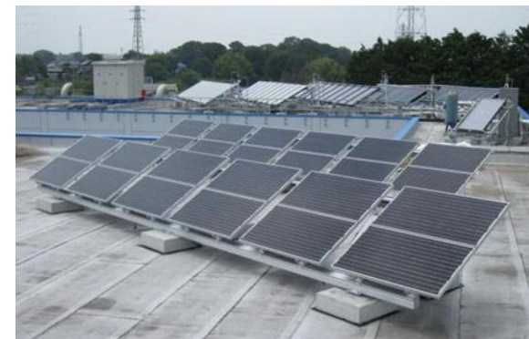
A solar hybrid panel (at the Hibiya Engineering Noda Research Center)
