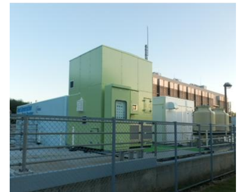
Modular data center
