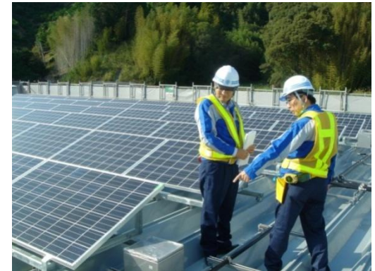
Expressway parking area solar power system for NEXCO Central
