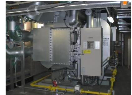
High-efficiency gas absorbing cold-hot water generator (Four Seasons Hotel Chinzanso)
