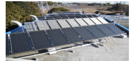
Solar thermal system demonstration test at the Noda Technology Research Center
