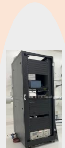
Increased per-rack heat generation due to ultra-high density
